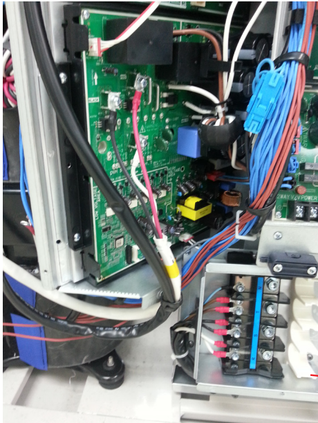
► Comp wire & valve,sensor wires fix by Holder wire.
