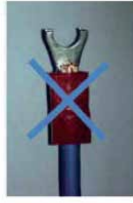
Terminal has been cut.
